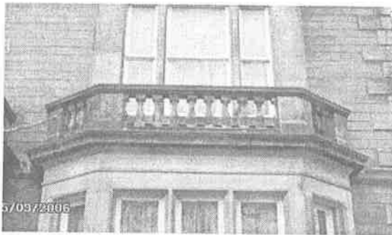
Figure 7. Soiled front balcony
